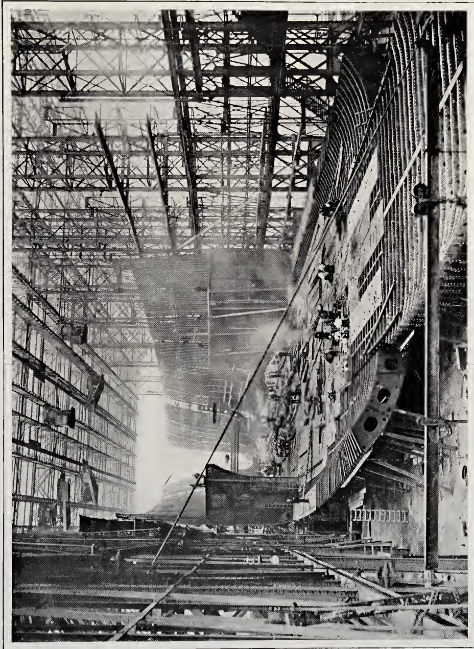
THE BUILDING OF THE "MAURETANIA." Showing Floor and part of Frames. From a Photograph. By permission of the Cunard Steamship Co.
